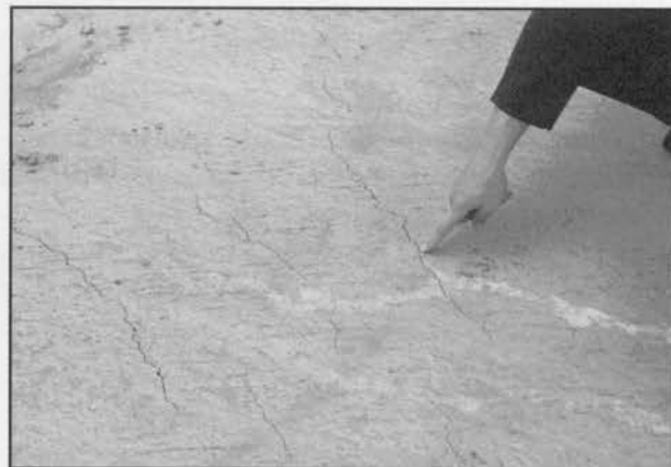
Plastic Shrinkage Cracks
